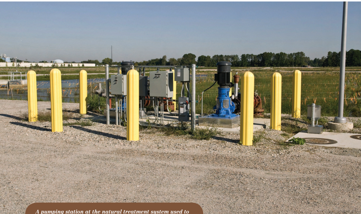
A pumping station at the natural treatment system used to pump effluent as needed during high flows.
